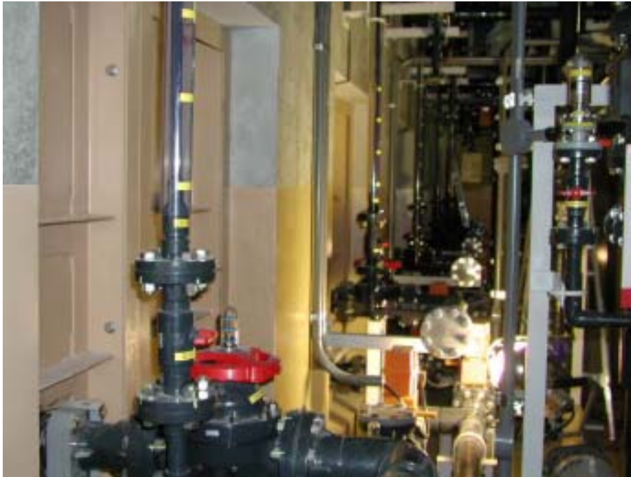
Electrolyte Tanks and Pipes
